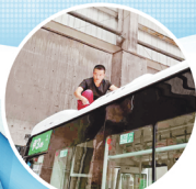
维修工常锐正在维修公交车空调
